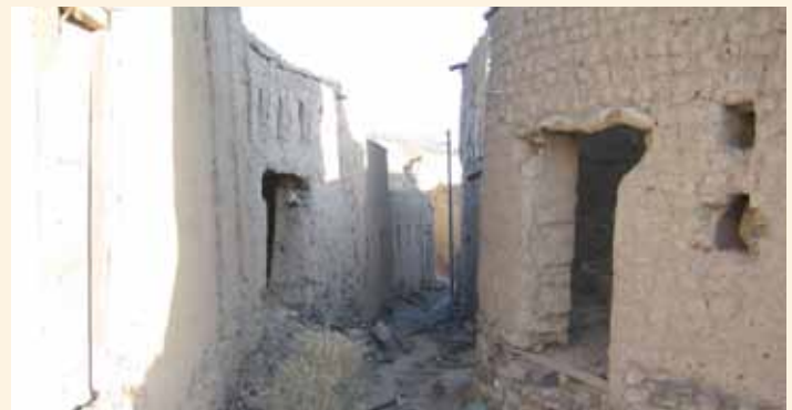
TOP Bahla's evocative mud-brick walls do not do well in the rainy season, and have been renovated continuously for a quarter of a century.
